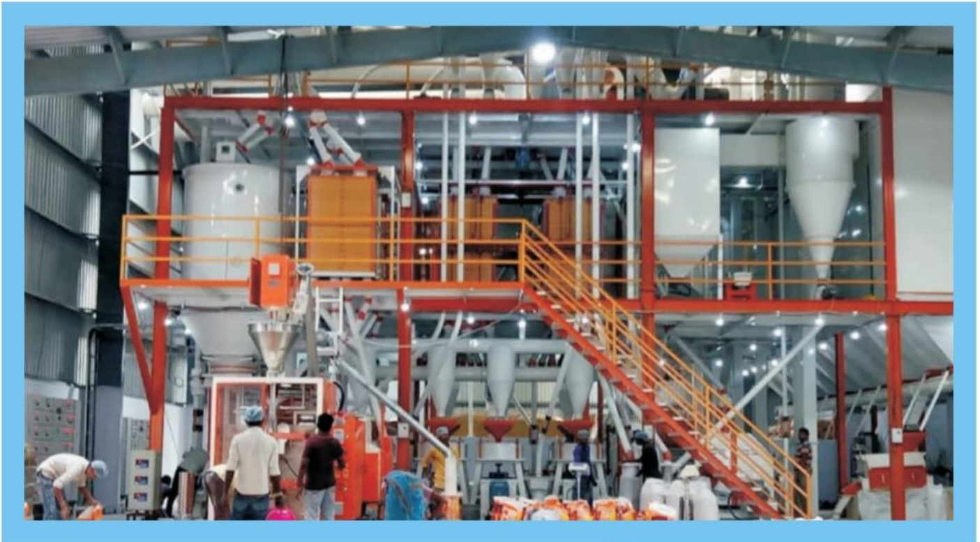
ATTA CHAKKI PLANT
